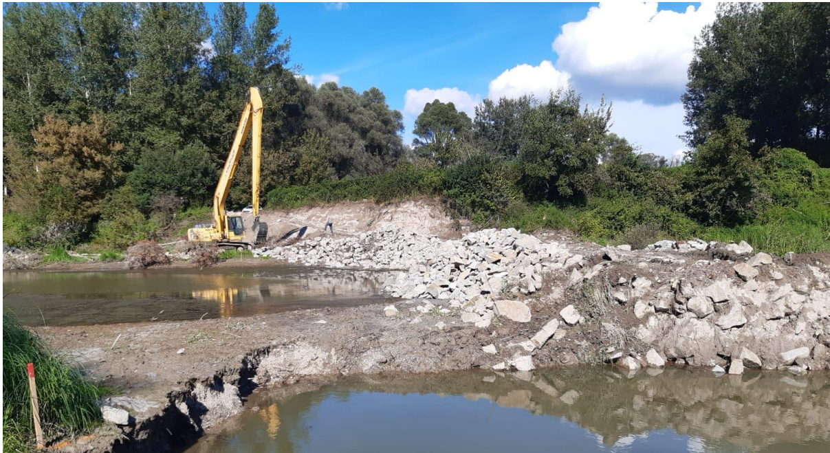
Work on removing of stone barriers in the basin of the Foki side arm (BROZ archive)
