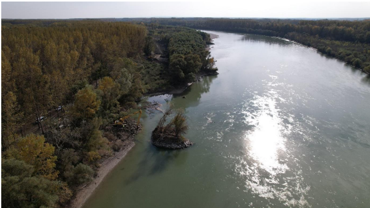
Work on removing of stone barriers in the basin of the Foki side arm (BROZ archive)
